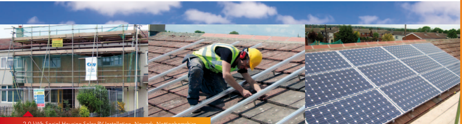
2.0 kWh Social Housing Solar PV Installation, Newark, Nottinghamshire.
