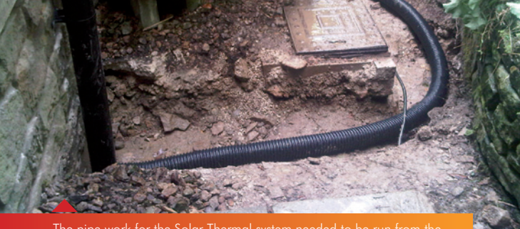
The pipe work for the Solar Thermal system needed to be run from the main loft space to a separate garage located away from the house.
