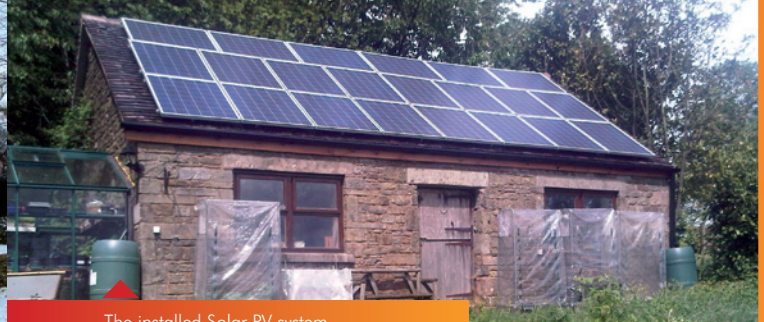
The installed Solar PV system.
