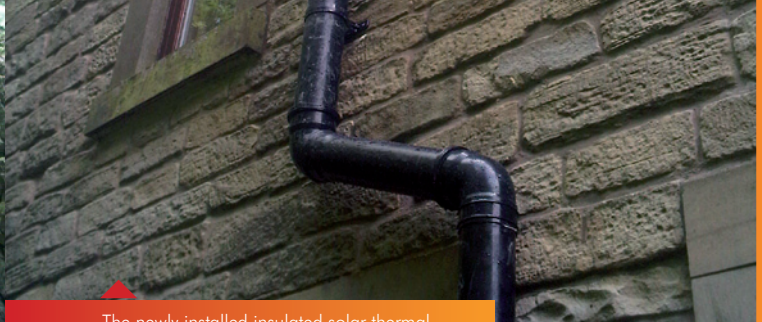
The newly installed insulated solar thermal pipe work within the plastic downpipe.
