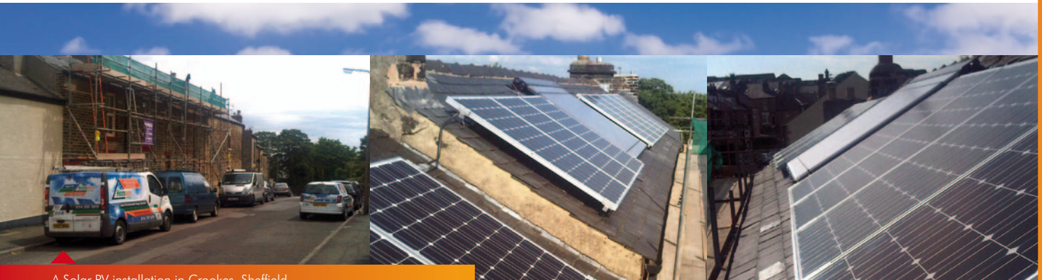
A Solar PV installation in Crookes, Sheffield.
