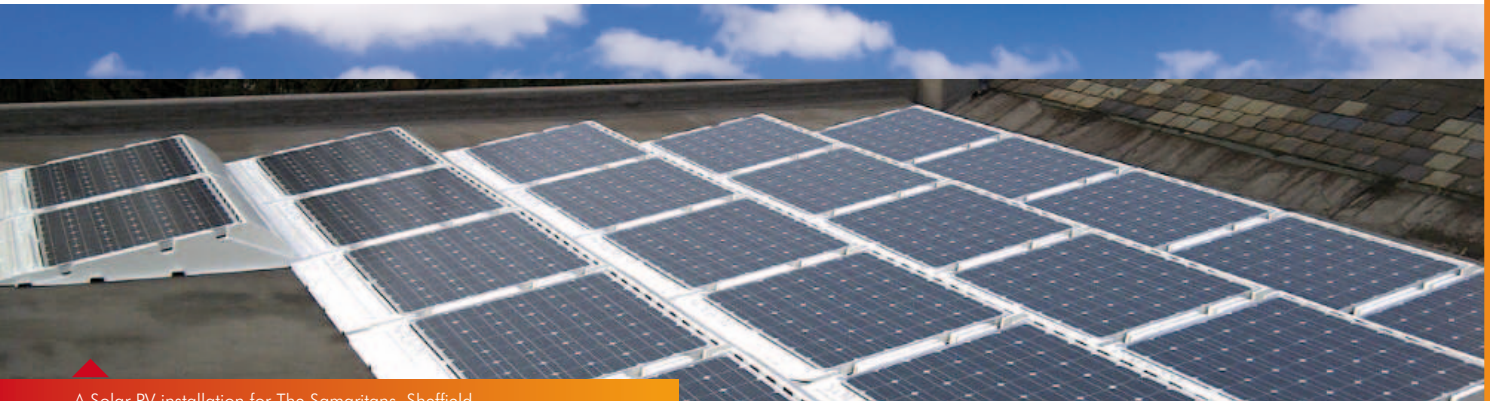
A Solar PV installation for The Samaritans, Sheffield.
